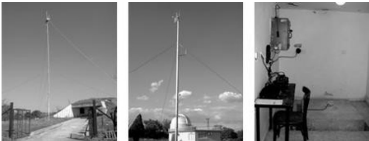
Fig. 2. Seismic stations Provardia, Avren and Roiak (ROA) — mast, antenna, radio-modem, lightning protection and the installed seismological equipment on ss Roiak and Avren — geophone as seismometer, DAS Reftek 130-01 lightning protection; height of the masts are correspondingly 25, 13 and 14 m
